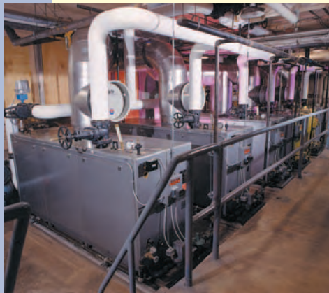
Six Bryan boilers replace two 300 HP boilers at Carver Senior High School, New Orleans, with six stage lead-lag system matching output to demand, for maximum economy.
